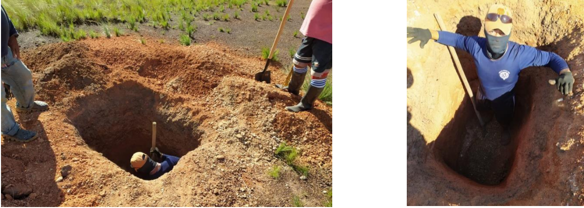
Figure 8. In trenches T01, T02, and T03 the trenches cut rock. Notice the white clay (kaolin) product of the weathering of the granite.
